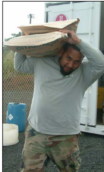
The crew hand-loads 50 lb bags of citric acid into the work truck.
